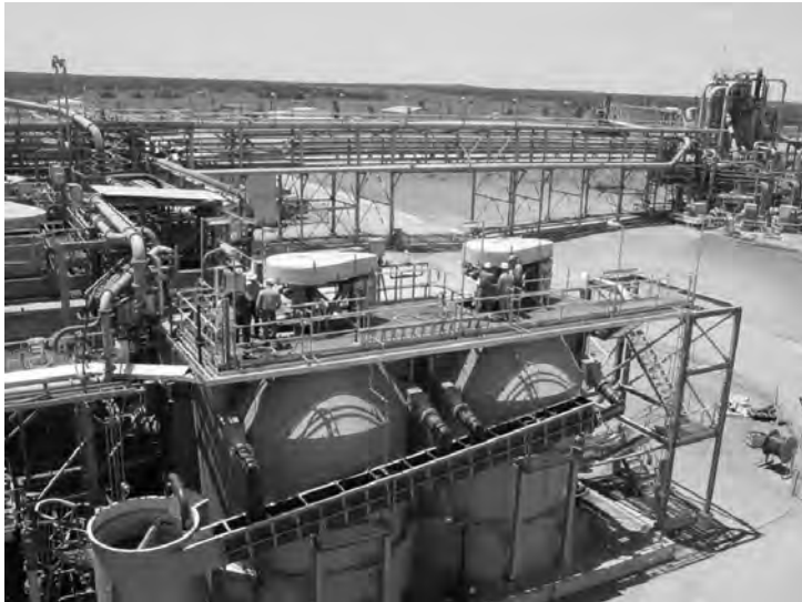
Fig. 1: Flotation cells used at Mt Keith (Western Australia) for nickel production (Reproduced with permission of BHP-Billiton.)
